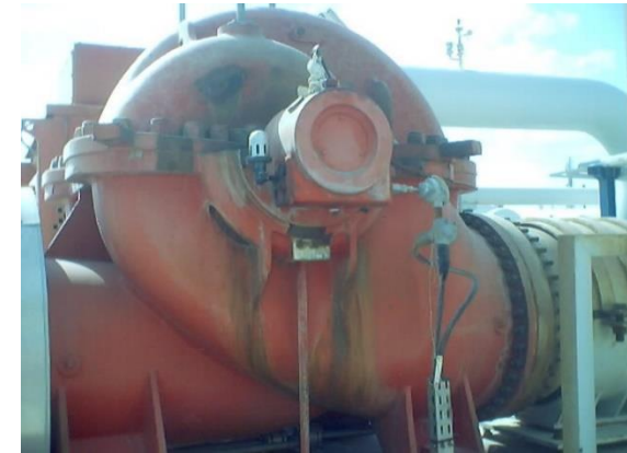
Pump in service after CMS -2000 installation by 18 months
