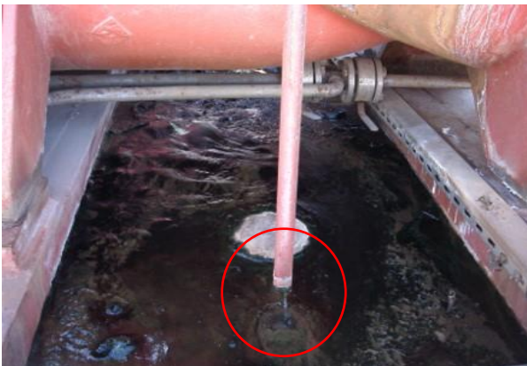
Pump leakage before installing CMS-2000
