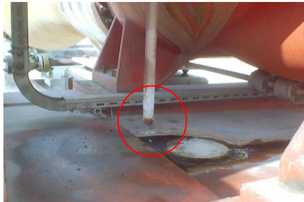
Pump leakage after installing CMS-2000
